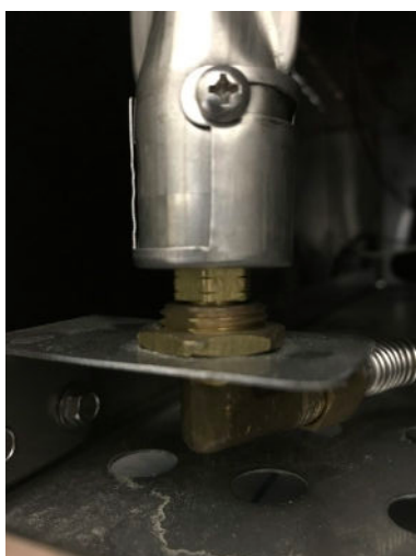
REAR BURNER PROPERLY SEATED
