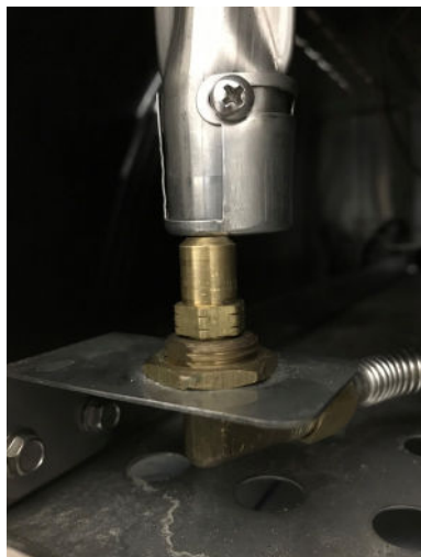
REAR BURNER NOT PROPERLY SEATED
