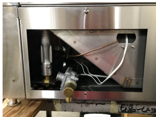
Rear Access Panel Removed
