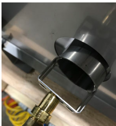
HEARTH BURNER NOT PROPERLY SEATED
