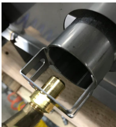
HEARTH BURNER PROPERLY SEATED
